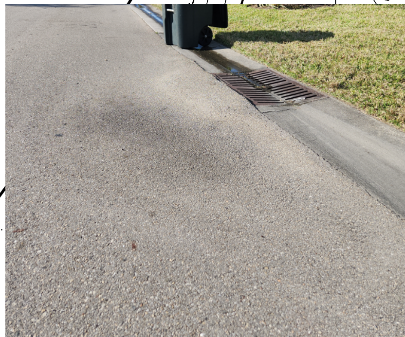
Loc.18: No depression in inlet. Major depression in pavement and minor depression in curbing around inlet (both sides). Crack in curbing by inlet (possible inlet lifting) (both sides), 1 panel each side.
