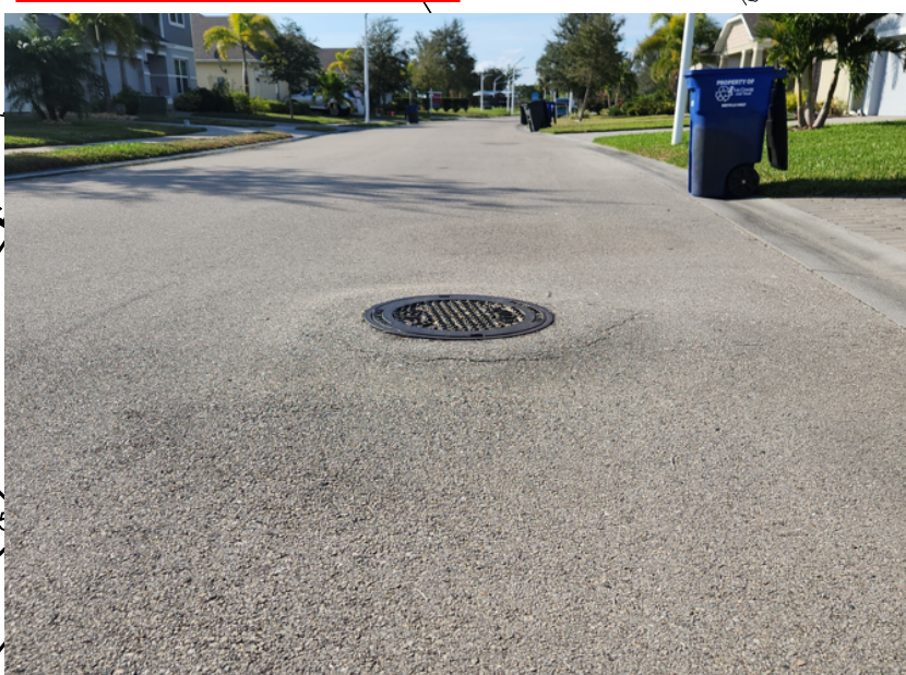
Pavement depression and cracking around MH
