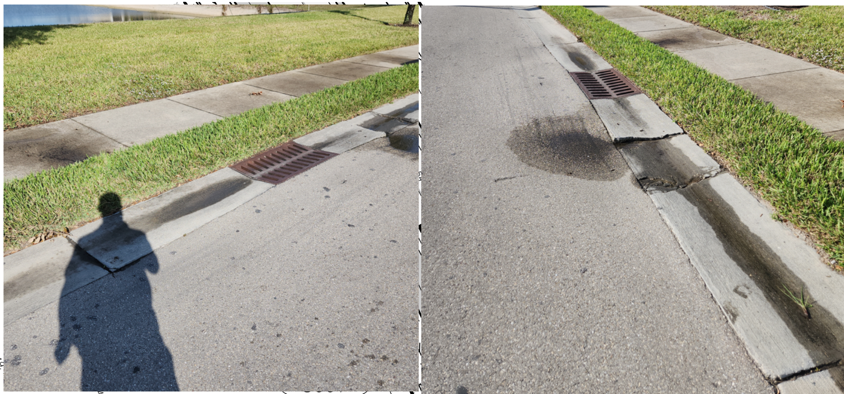
Loc.15: No depression in inlet. Major depression in pavement and in curbing around inlet (both sides). Crack in curbing (both sides), 1 panel each side ~ 18LF.
