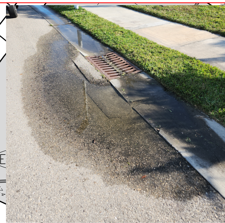
Loc.17: No depression in inlet. Major depression in pavement and 2 asphalt patches are lifting. Major curbing depression around inlet (both sides). Crack in curbing (both sides), 1 panel each side ~ 16LF.
