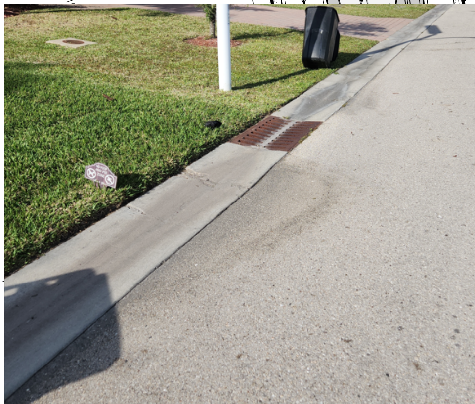
Loc.14: No depression in inlet. Minor depression in pavement and in curbing around inlet (both sides). Crack in curbing (both sides), 1 panel each side ~ 20LF.
