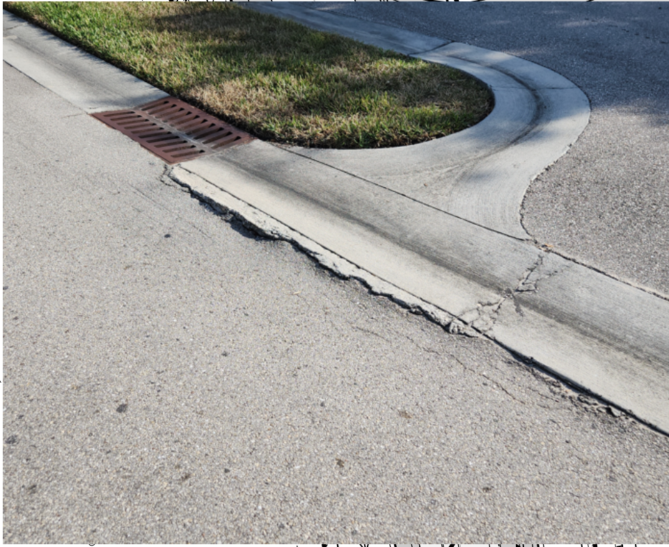
Loc.16: No depression in inlet. Major depression in pavement abutting curb (W side). Crack in curbing (W side), 1 panel ~ 10LF.
