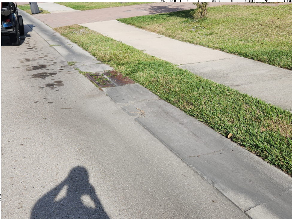
Loc.13: No depression in inlet, filter fabric still in. Minor depression in pavement and major depression in curbing (both sides). Crack in curbing (both sides), 1 panel each side ~ 20LF.
