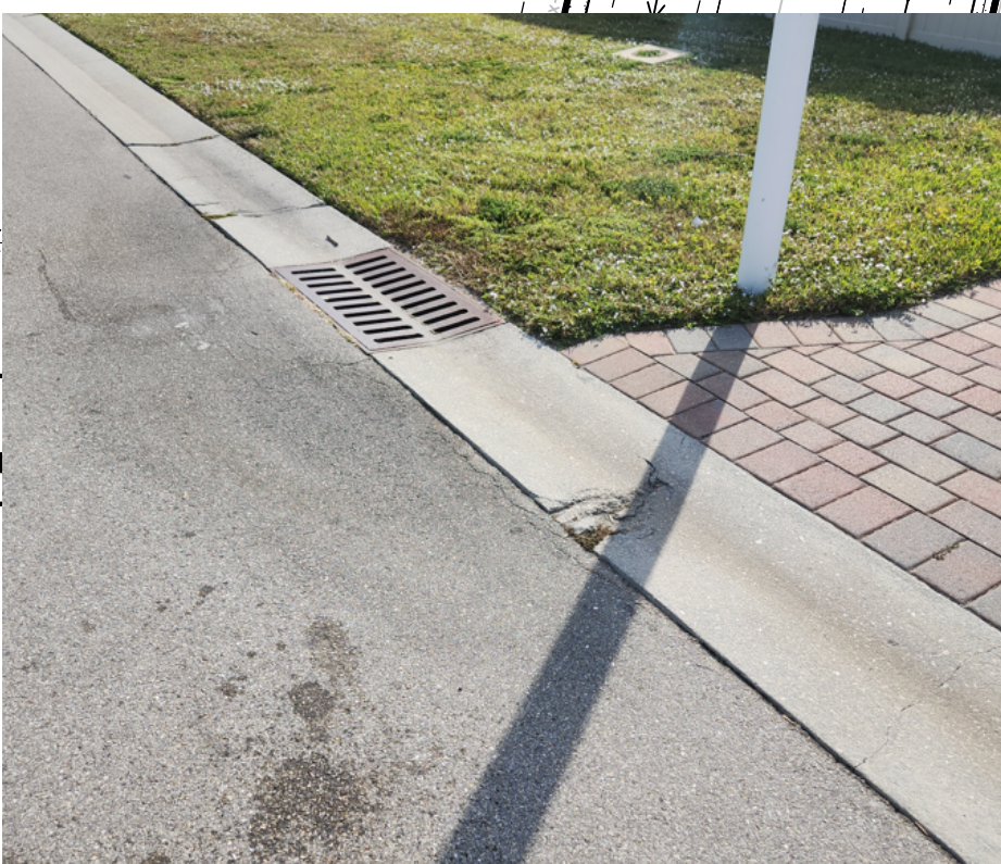
Loc.11: No depression in inlet. Noticeable depression in pavement and curbing around inlet. (both sides). Crack in curbing (both sides), 1 panel each side ~ 18LF.
