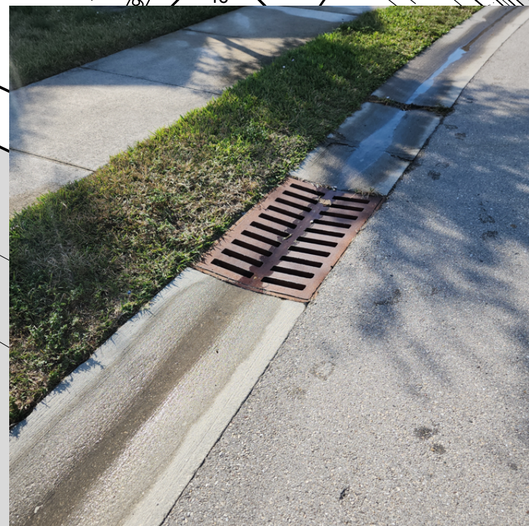
Loc.19: No depression in inlet. Minor curbing depression (W side). Crack in curbing (W side), 1 panel each side ~ 10LF.
