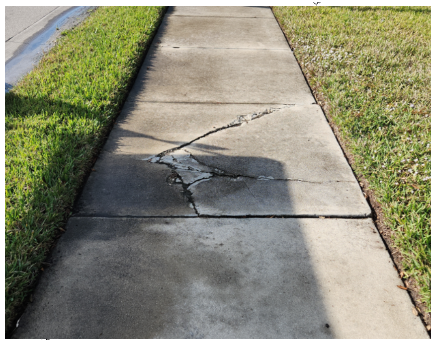
Sidewalk panel lifting and cracked
