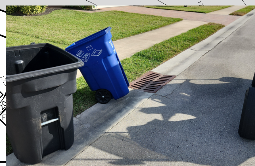
Loc.12: No depression in inlet. Noticeable depression in pavement with pavement cracking. minor curb depression (N side). Crack in curbing (N side), 1 panel ~ 8LF.
